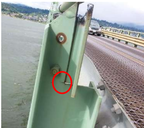
Figure 3. Span 16, P11 tear in coped web of post.
