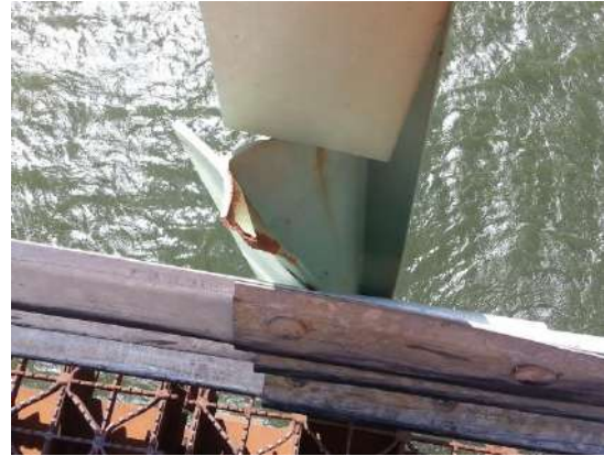
Figure 5. Span 17, P32 significant post deformation
