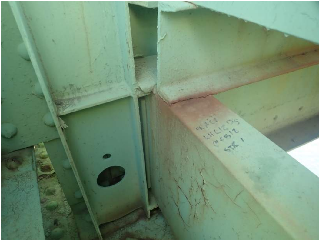
IM06645_A7: Crack in Sub-Stringer to Stringer 1 at Floorbeam 11 in Span 11
