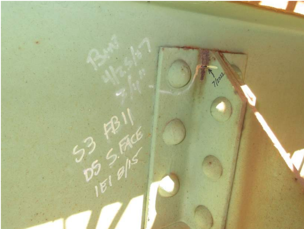
IM06645_D3: 1" Crack at Knee Brace at Floorbeam 11 in Span 3
