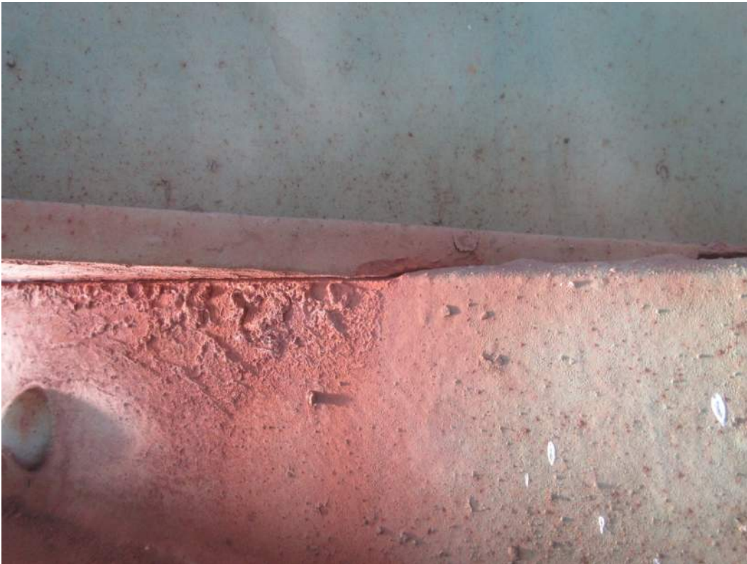
IM06645_B1: Lateral Bracing Rubbing against Stringer 2 in Span 11 Resulting in Section Loss
