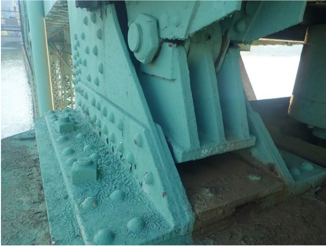
IM06645_E4: 3/4" Gap Beneath Span 11 Pier 12 DS Bearing
