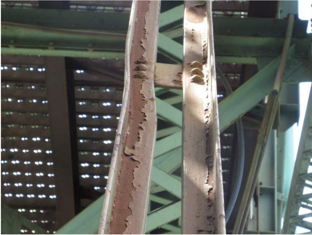
IM06645_C4: 1" over 2' Out of Plane Bending at U2L3 of Span 12 DS
