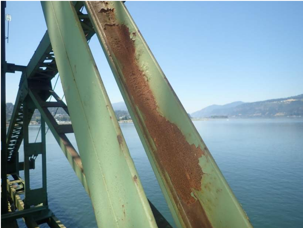
IM06645_B7: Typical Paint Failure and Surface Corrosion on Truss Diagonal Members
