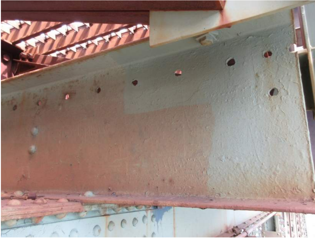
IM06645_D4: Torch Cut Holes in Floorbeam 4 of Span 12
