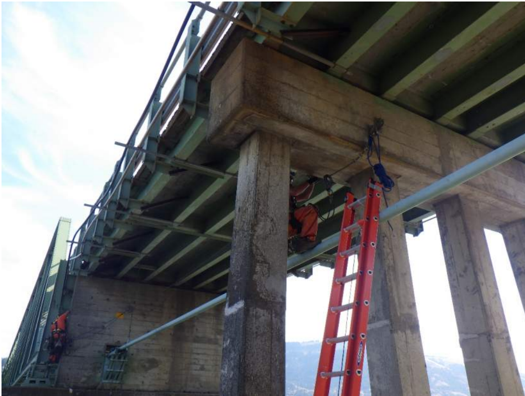
IM06645_D9: Bent and Leaning Column 1 at Pier D, Sealed Horizontal Cracks All Columns
