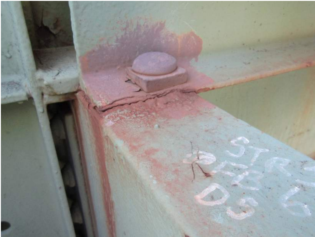
IM06645_A9: Crack in Sub-Stringer to Stringer 1 at Floorbeam 6 in Span 11
