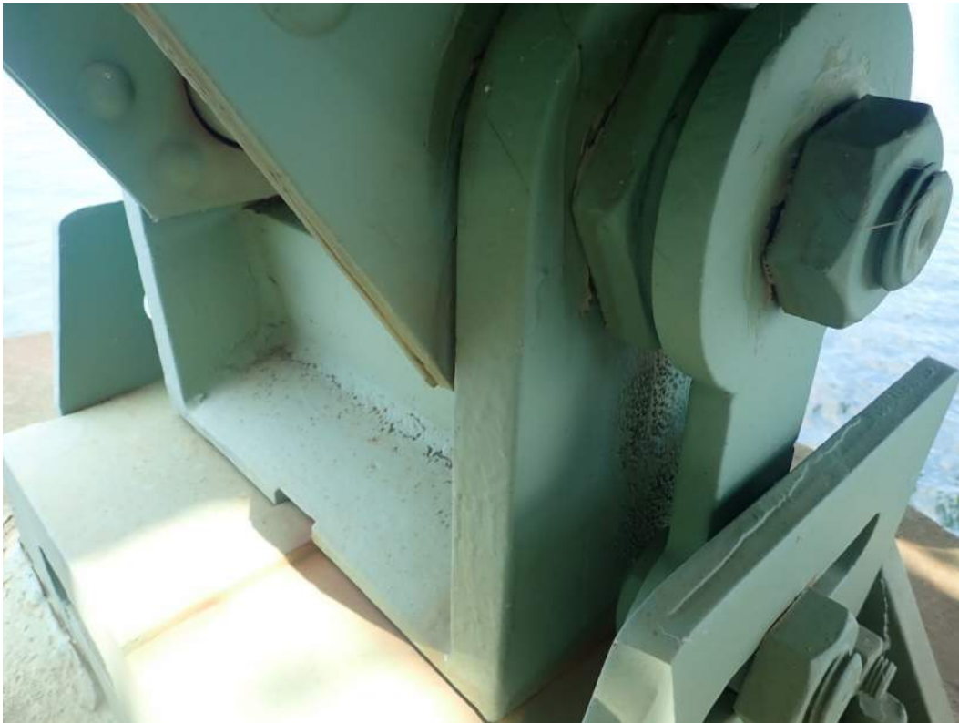
IM06645_E3: Typical Pitting on Rocker Bearing
