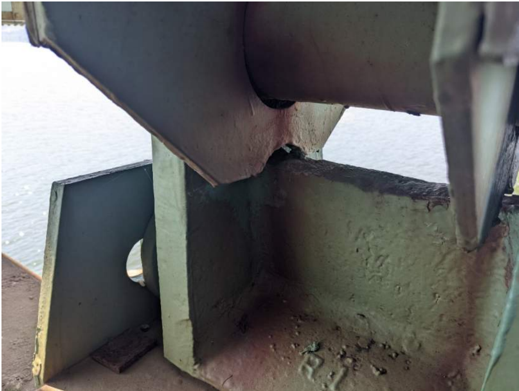
IM06645_E7: Typical Repair of Previously Identified Vertical Gussets Bearing on Rocker Stiffener
