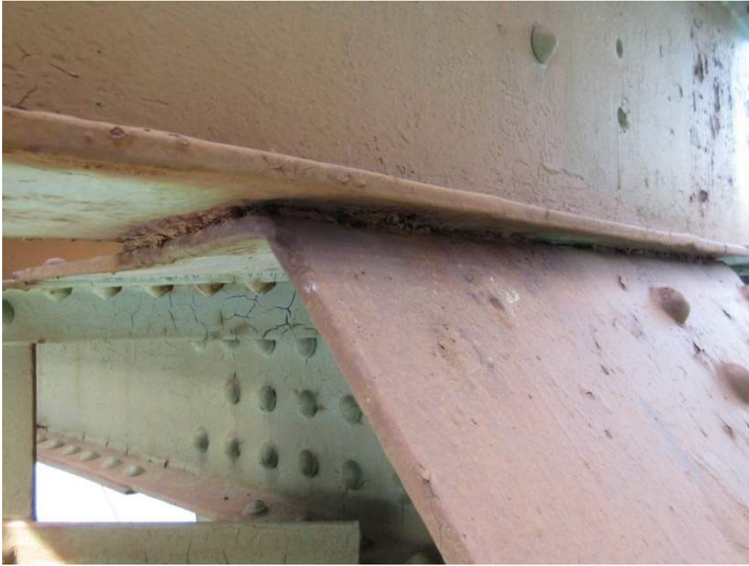
IM06645_C0: 3/8" Pack Rust between Floorbeam and Panel Point U10 in Span 12 DS
