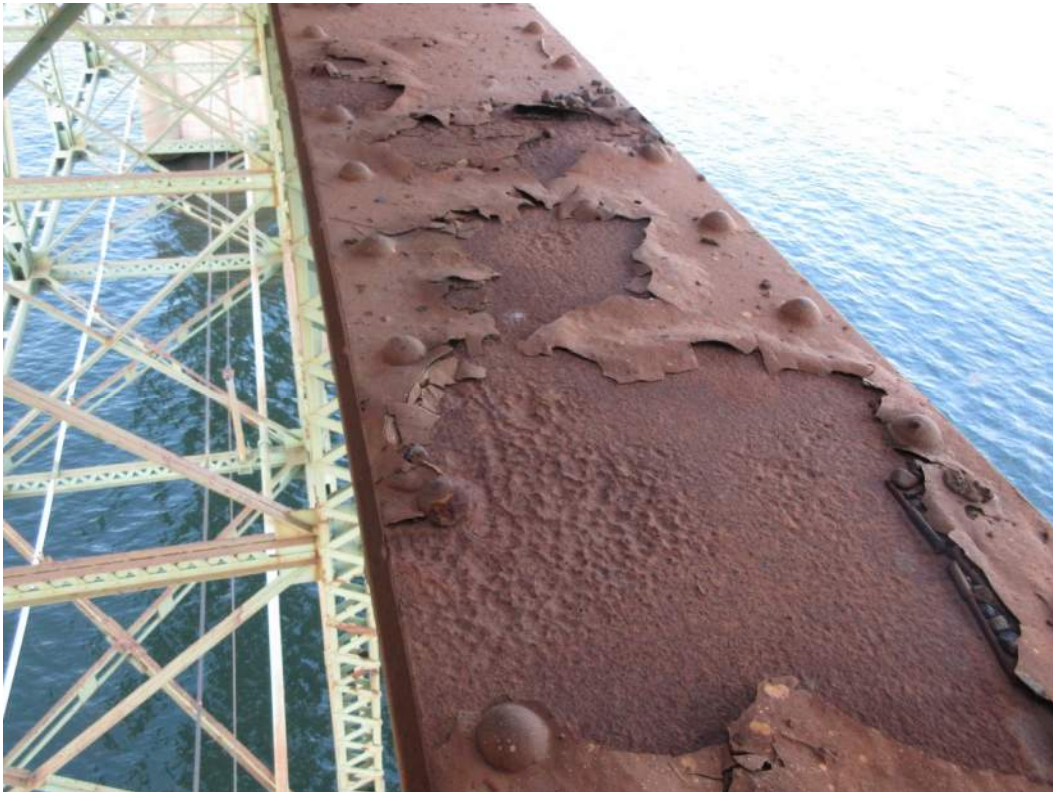
IM06645_B9: Paint Failure and 1/8" Pitting on U7U8 Top Chord of Span 8
