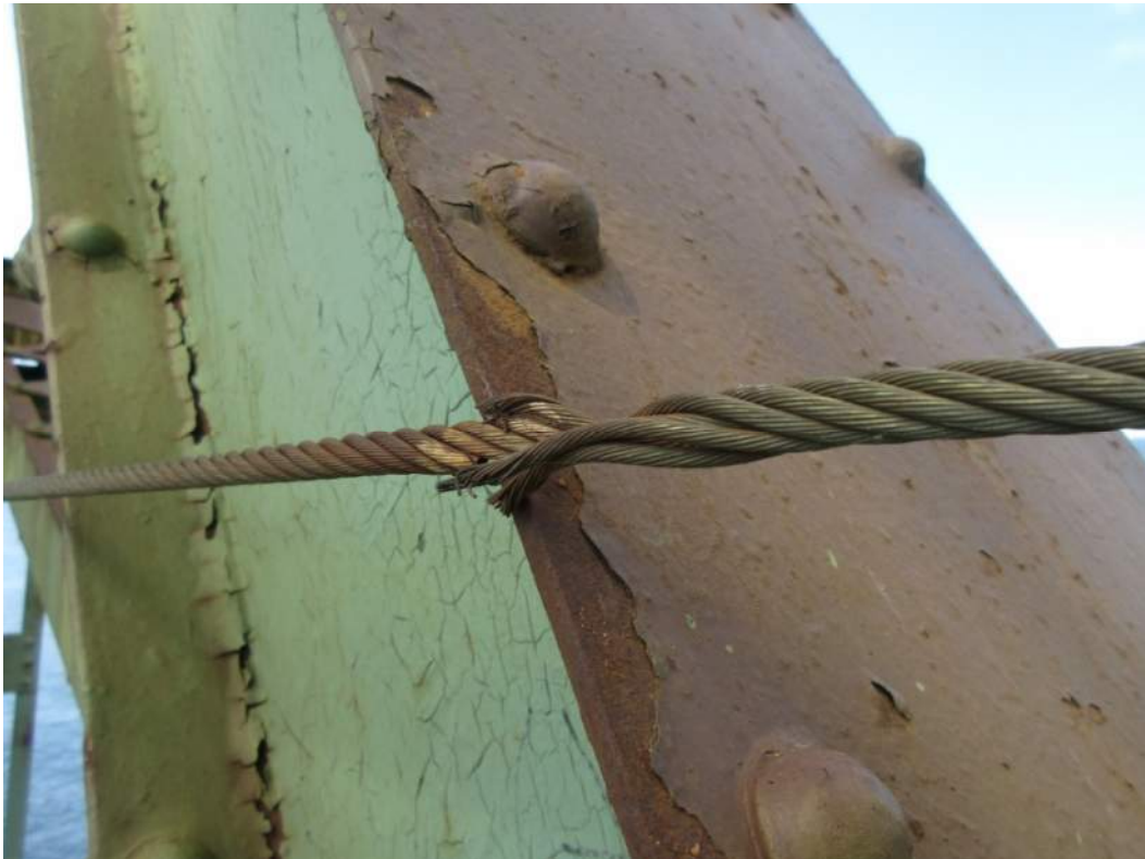
IM06645_F3: Broken Cables of Old Lifeline in Span 12 and 13
