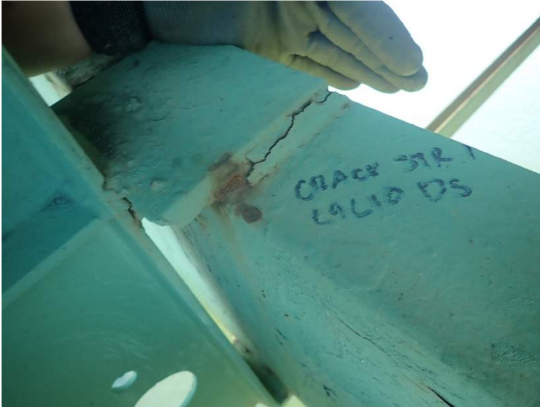
IM06645_A8: Crack in Sub-Stringer to Stringer 1 at midbay of L9L10 in Span 11
