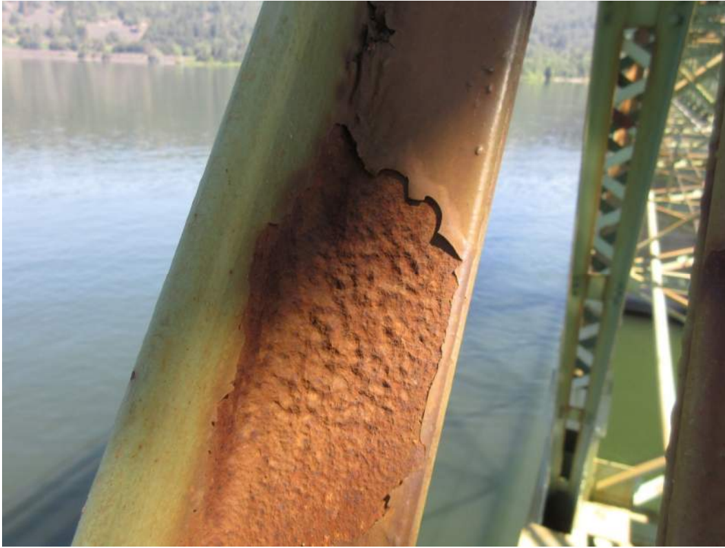
IM06645_B8: 1/8" Pitting on L5U6 Diagonal of Span 6 DS
