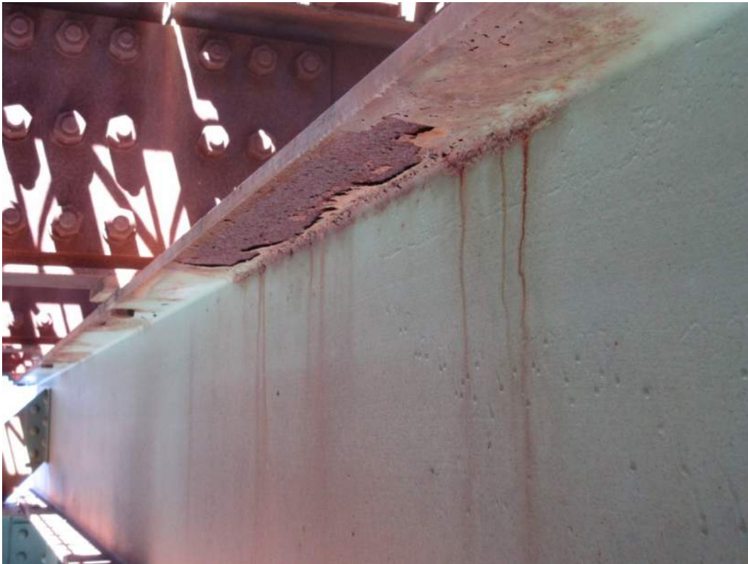
IM06645_C9: Typical Flaking Paint, Surface Corrosion, and Staining on Floorbeam
