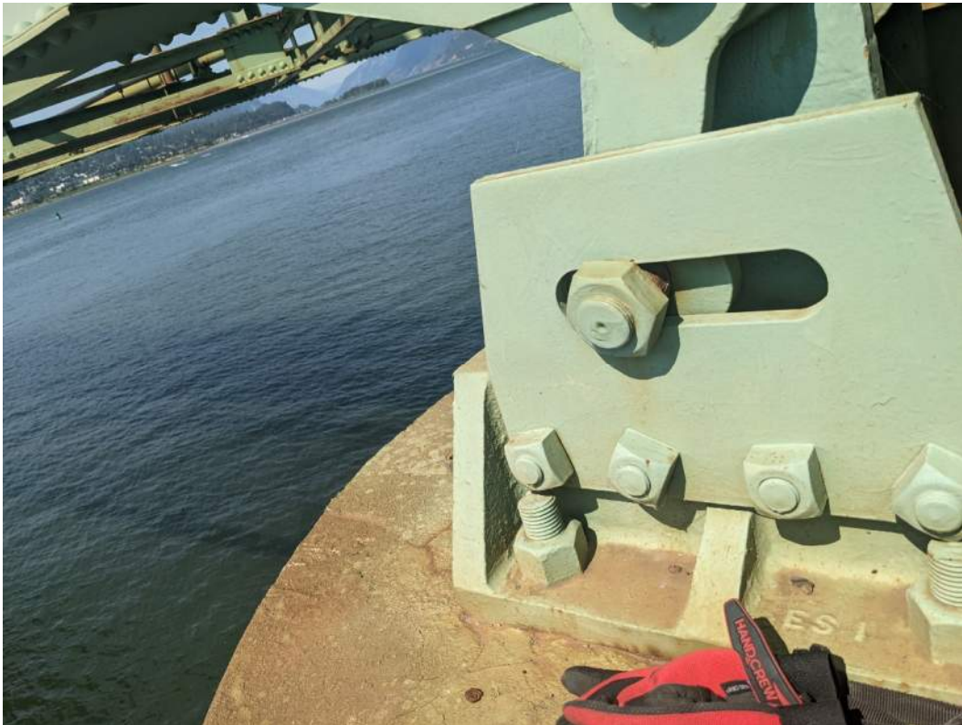
IM06645_E5: Typical Jammed Anchor Link at Bearing
