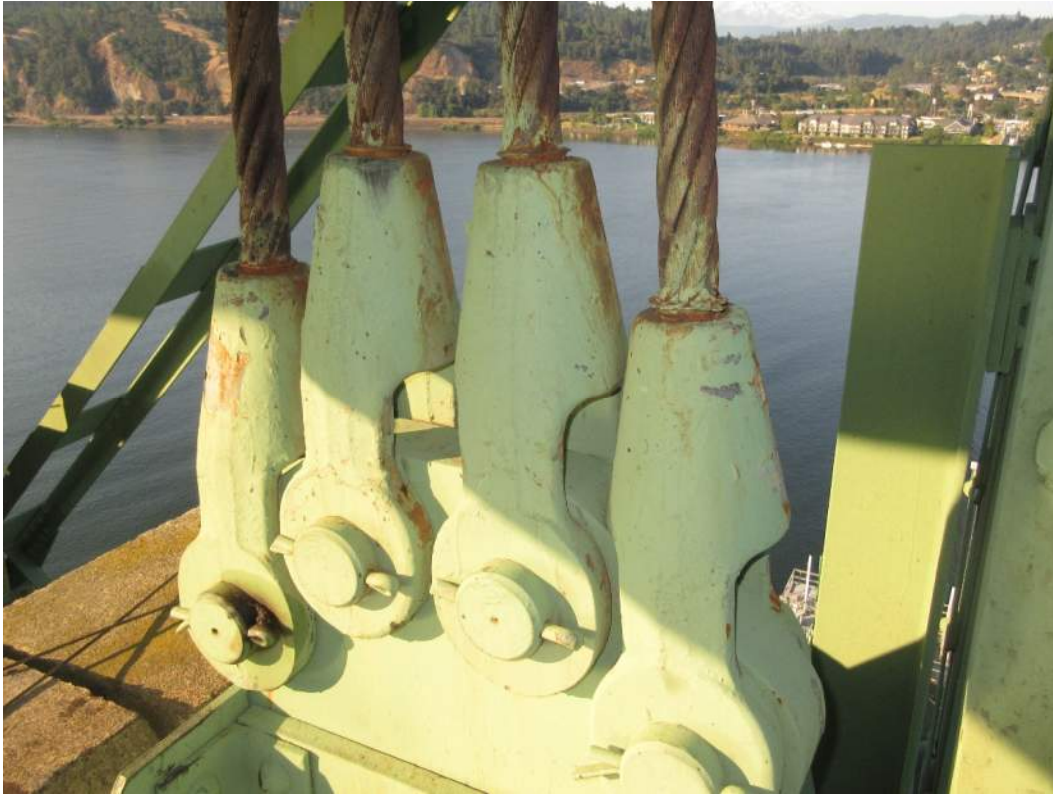
IM06645_F0: Span 11 Lifting Cables Pulled Out 3/8"
