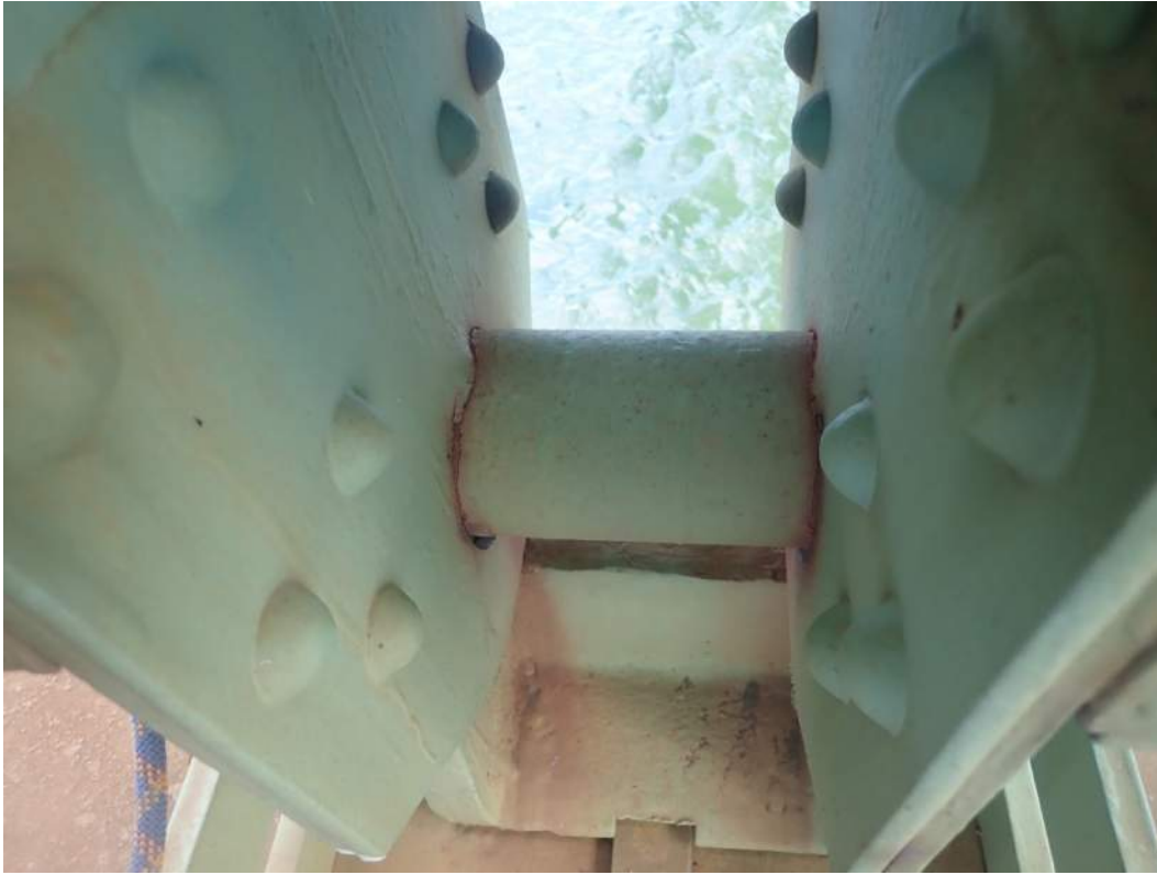
IM06645_E2: Crushed Vertical Gusset Plates at Span 3 Pier 3 DS Bearing
