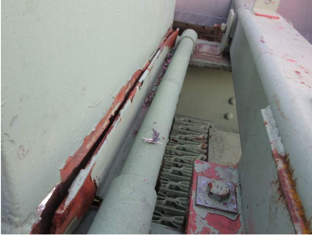
IM06645_F2: Broken Weld at Lift Pulley Covers
