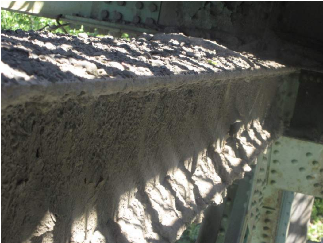
IM06645_B5: Heavy Debris Accumulation in Span 19
