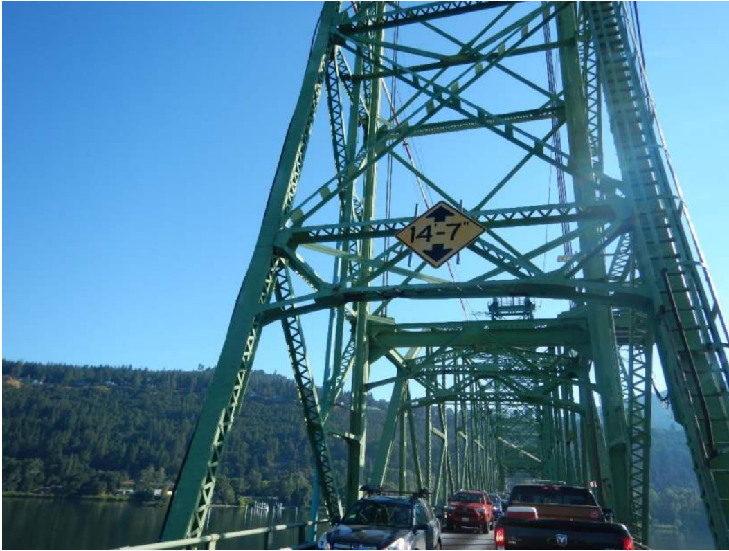
IM06645_C8: Impact Damage to Portal Bracing at Pier 11
