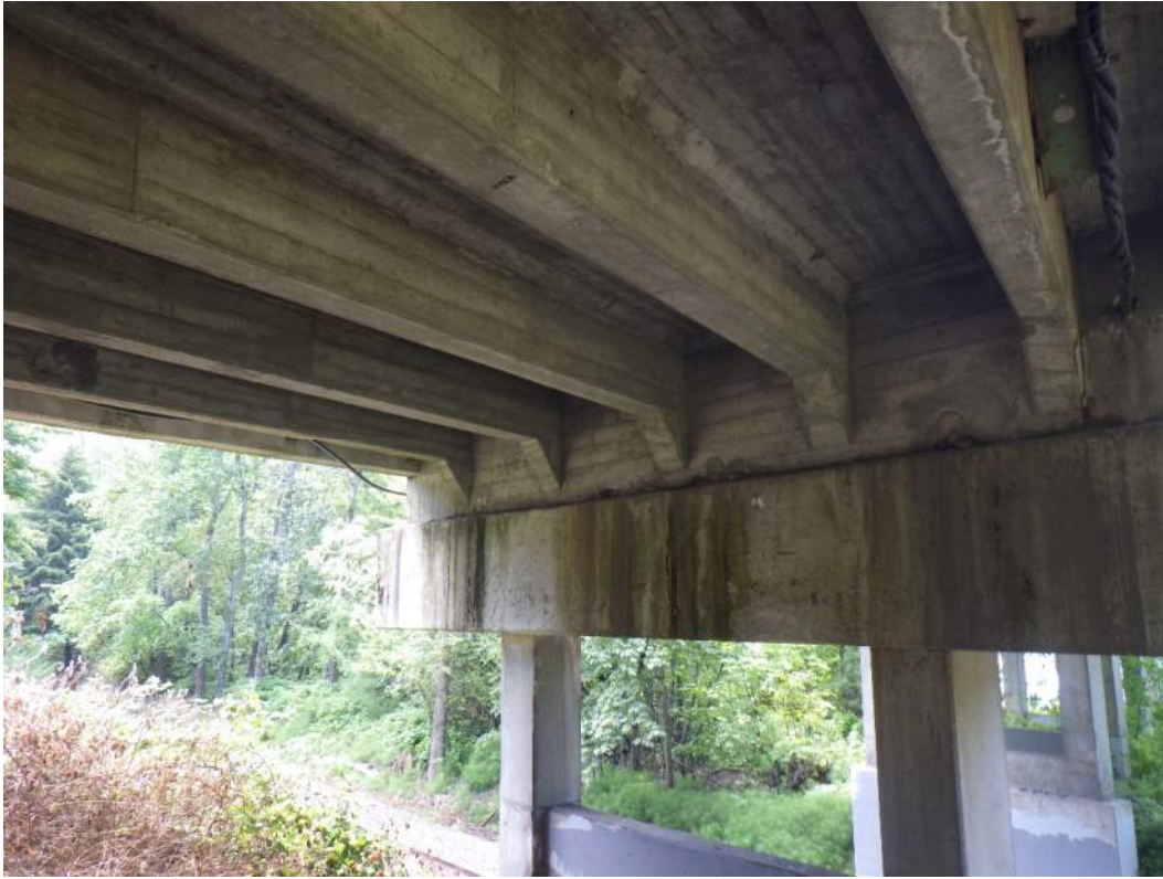
IM06645_A6: Spalls in Pier 27 End Diaphragm
