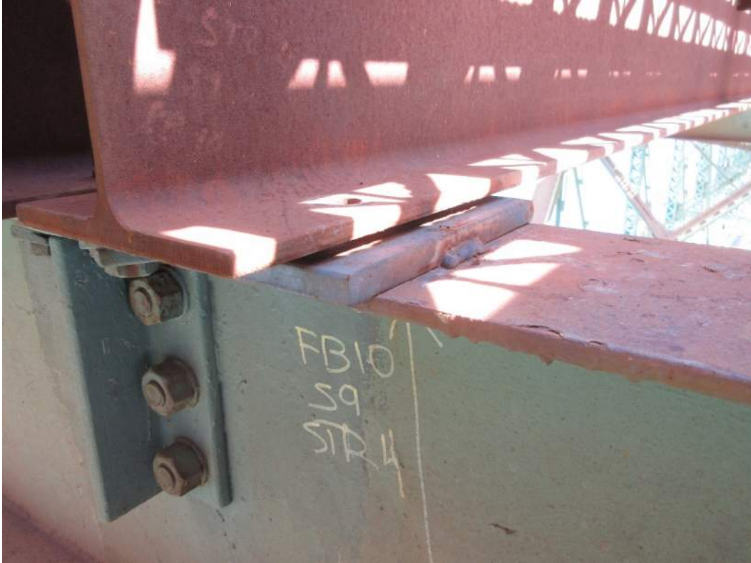
IM06645_B4: Bearing Gap at Stringer 4 at Floorbeam 10 in Span 9 with Broken Tack Weld
