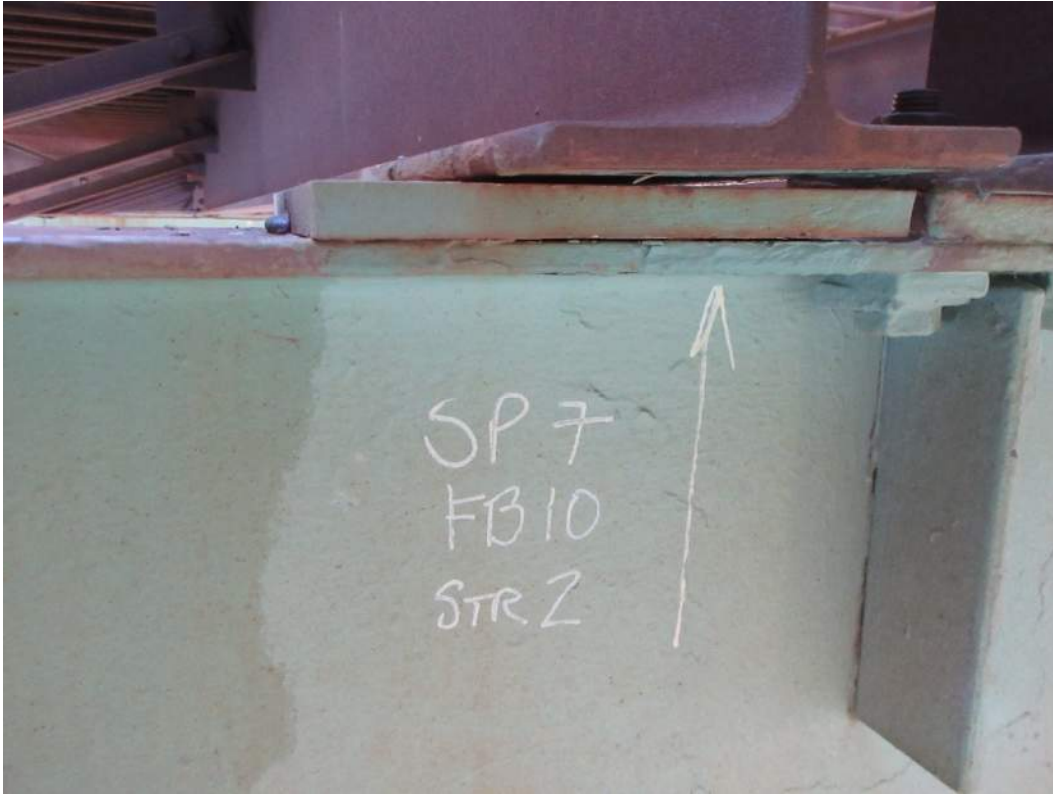
IM06645_B2: Minor Rotational Distortion and Bearing Gap at Stringer 2 at Floorbeam 10 in Span 7
