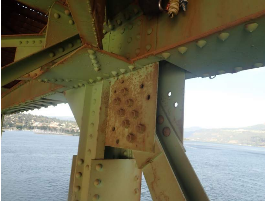
IM06645_D6: Typical Freckled and Surface Corrosion on Upper Gusset Plates
