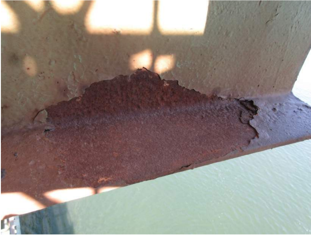
IM06645_D0: Pitting on Bottom Flange of Floorbeam 4 in Span 4
