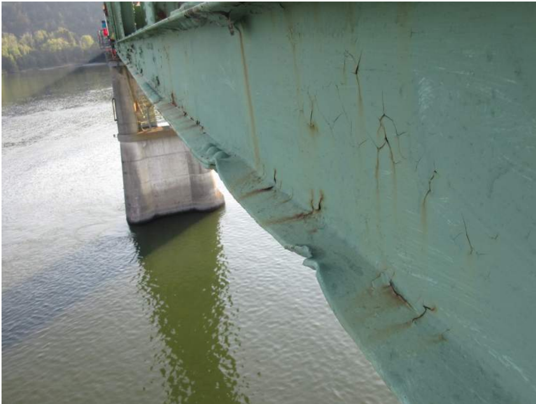
IM06645_C5: Collision Damage on L4L5 of Span 11 DS
