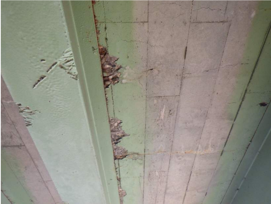
IM06645_A4: Spalls Adjacent to Girder Top Flange in Deck Soffit of Spans D and E
