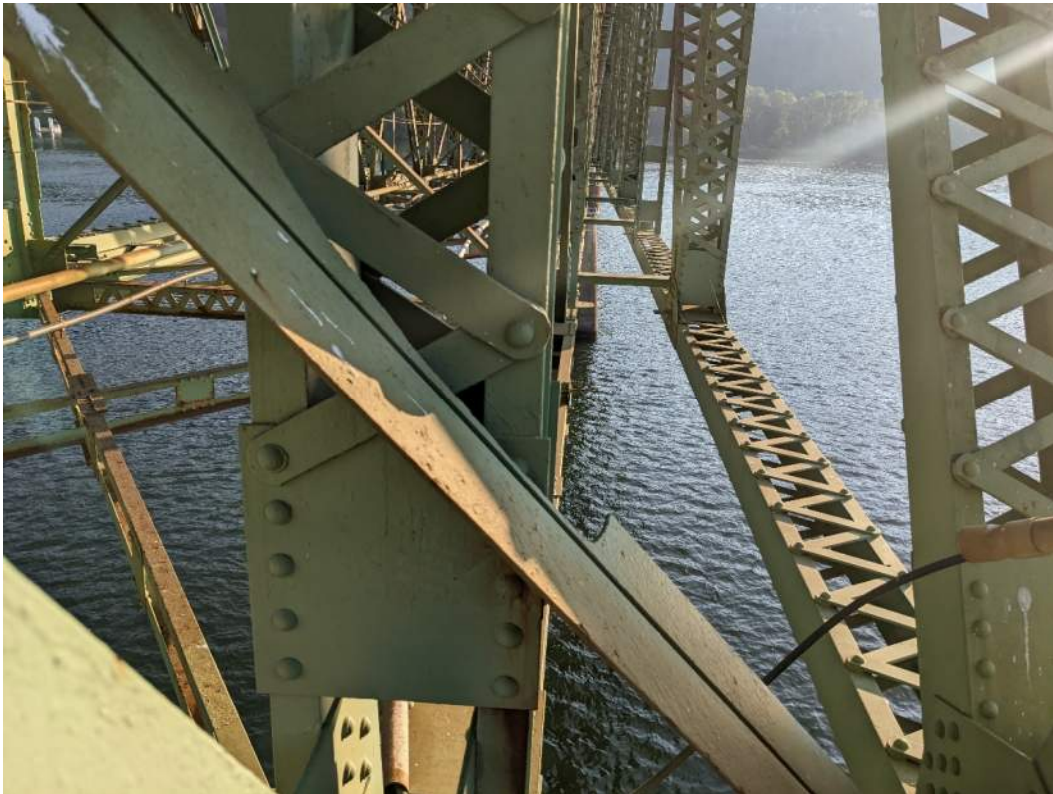
IM06645_C7: Sway Bracing Flange Cut at Panel Points L2 (US and DS) of Span 12
