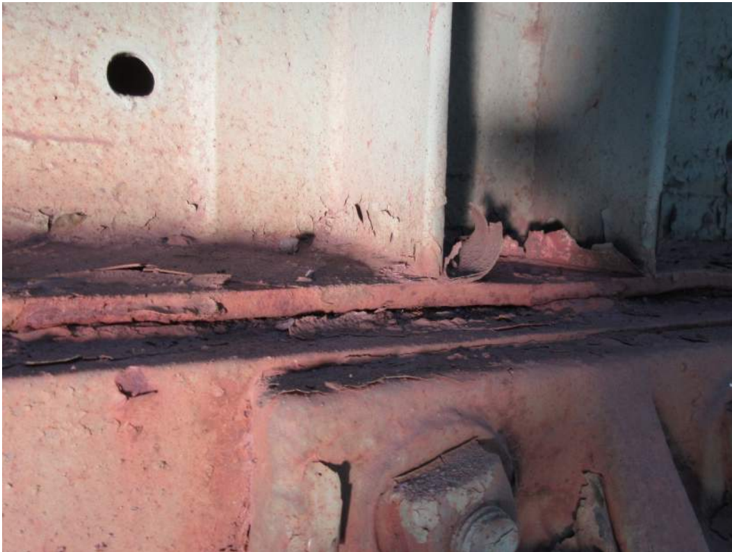
IM06645_D1: Pack Rust and Broken Tack Welds at Floorbeam 0 in Span 11
