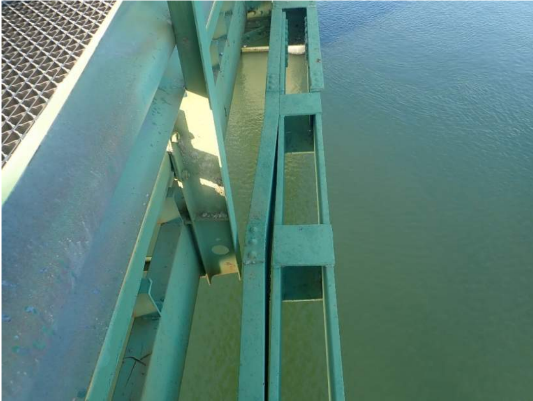
IM06645_C6: Repair due to Collision Damage at L7L8 of Span 11 DS
