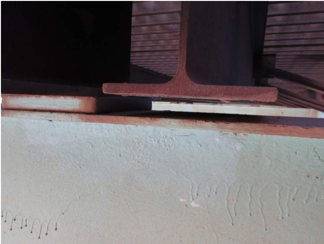
IM06645_B3: Missing Bearing Plate at Stringer 2 at Floorbeam 1 in Span 9
