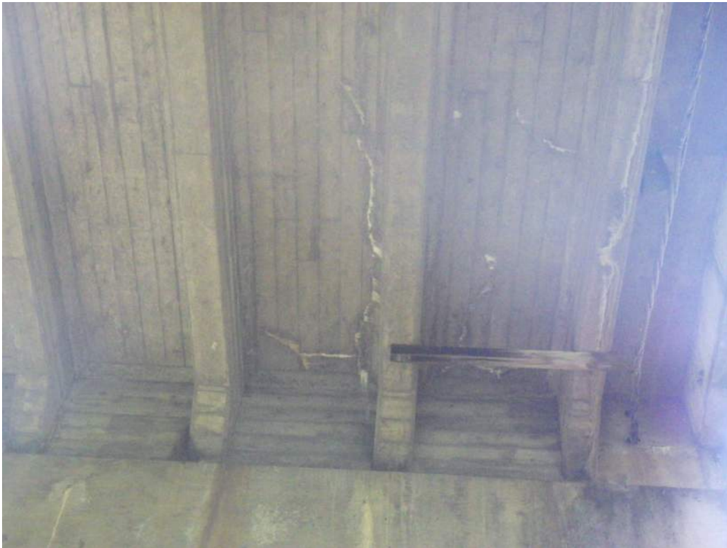
IM06645_A5: Longitudinal Cracks and Efflorescence in Span 21
