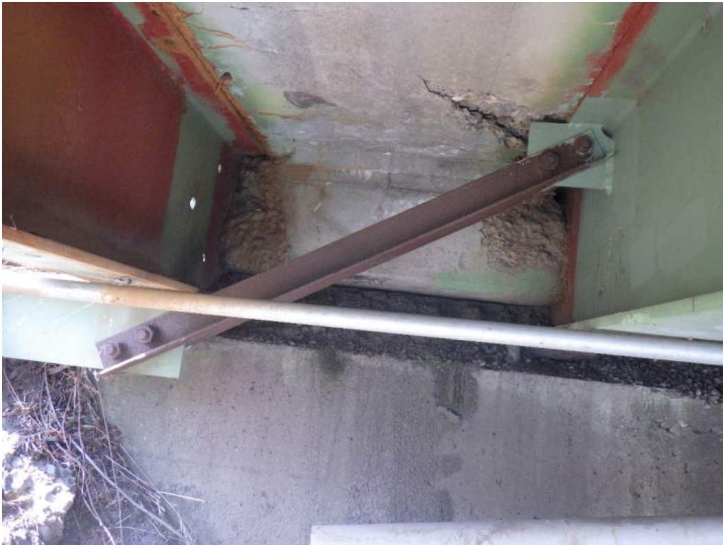
IM06645_A3: Spall and Delamination in Span E Soffit and Pier E End Diaphragm
