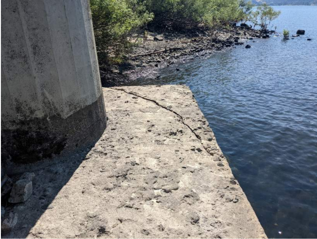
IM06645_E0: Pier 20 Exposed Spread Footing and Crack at Southeast Corner
