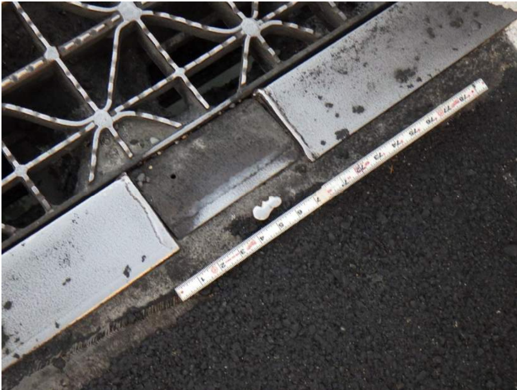
IM06645_E1: 7" Broken Section of Armored Header at Pier 20
