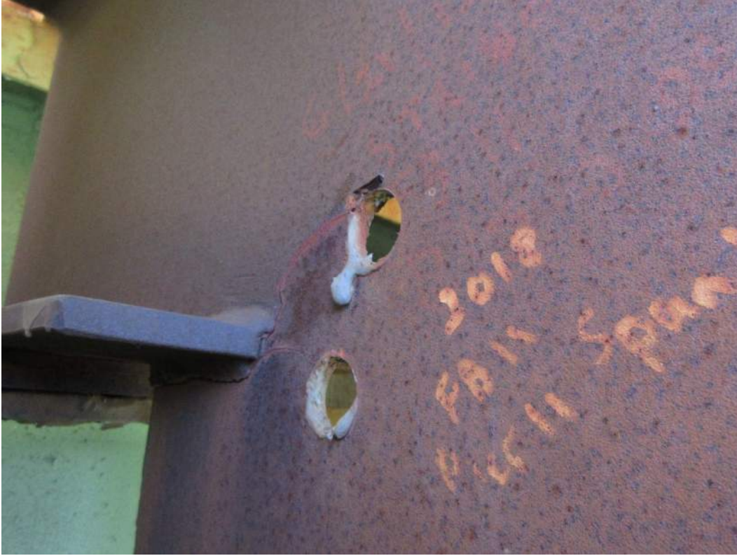
IM06645_B0: Arrested Cracks in Stringer 1 at Floorbeam 11 in Span 10
