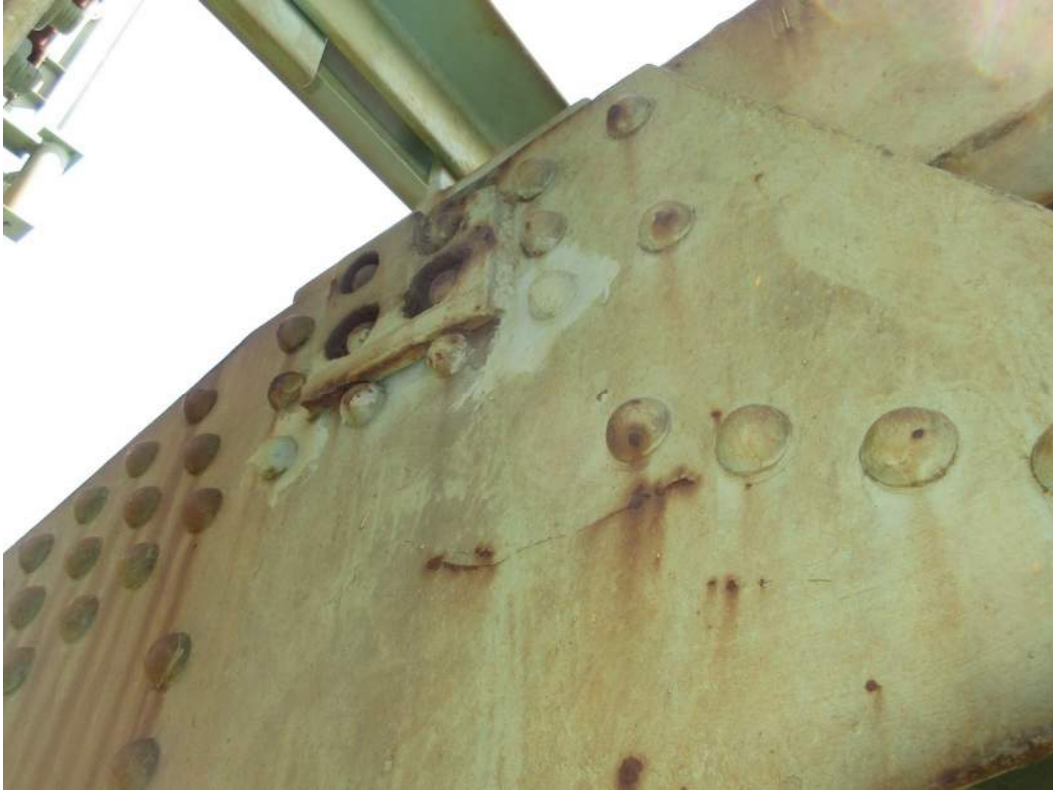
IM06645_C2: Remnants of Auxiliary Truss Upper Connection at Panel Point U10 of Span 12 DS
