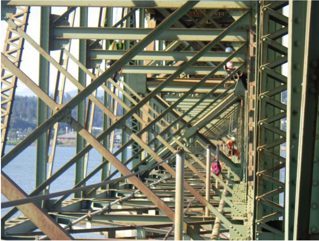
IM06645_B6: Typical Paint Condition and Surface Corrosion on Truss Spans
