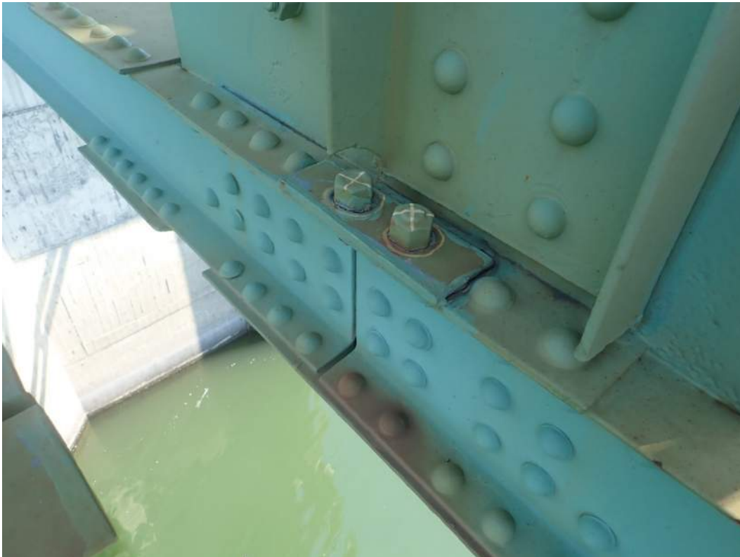
IM06645_C1: Remnants of Auxilary Truss Lower Connection at Panel Point L10 of Span 10 DS
