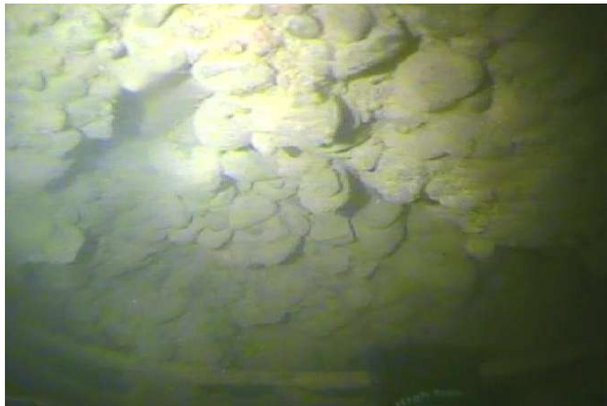
Figure 2 Pier 6 upstream column
