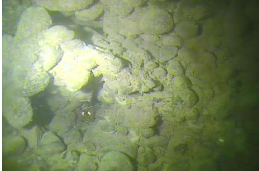
Figure 1 Pier 8 south side web rock pockets
