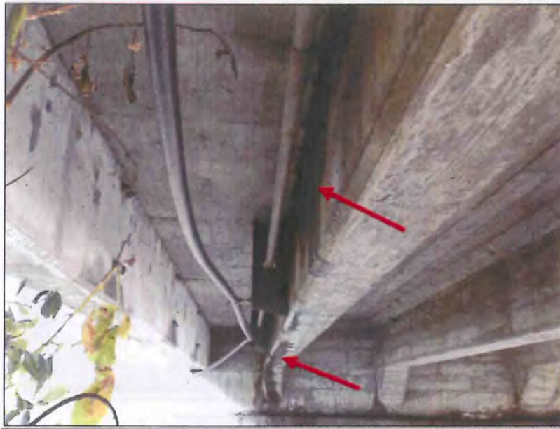
Figure 2: Moisture through the Cold Joint
