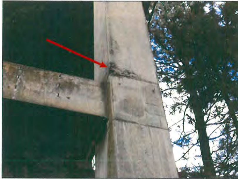
Figure 4: Rock pocket in Column
