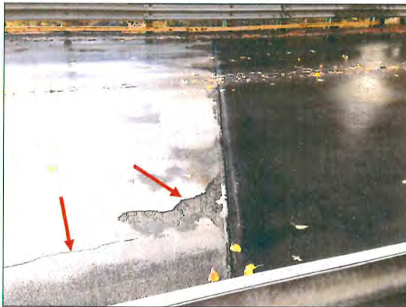
Figure 1: Cracks and Spalls on the Concrete Overlay System (North Approach Structure)
