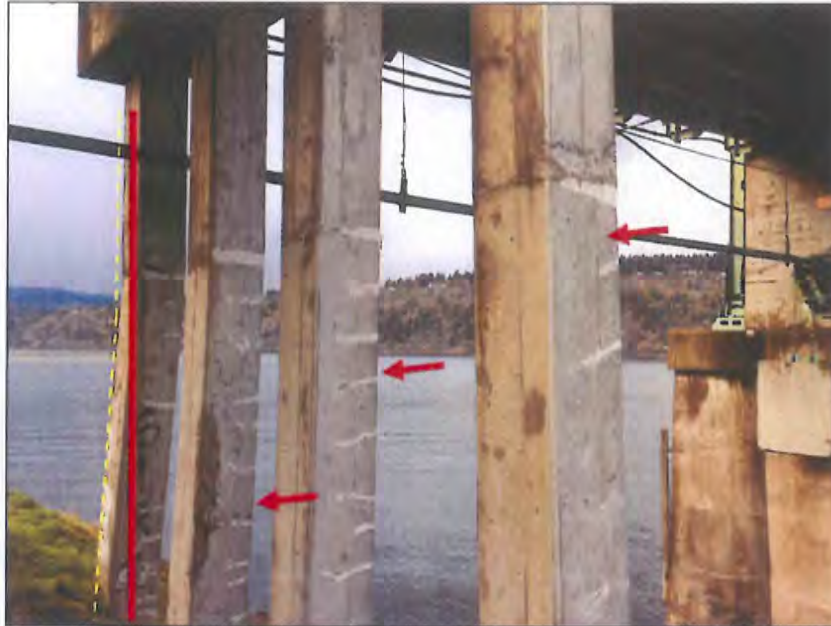
Figure 5: Bent 2 flexural cracking and deflection
