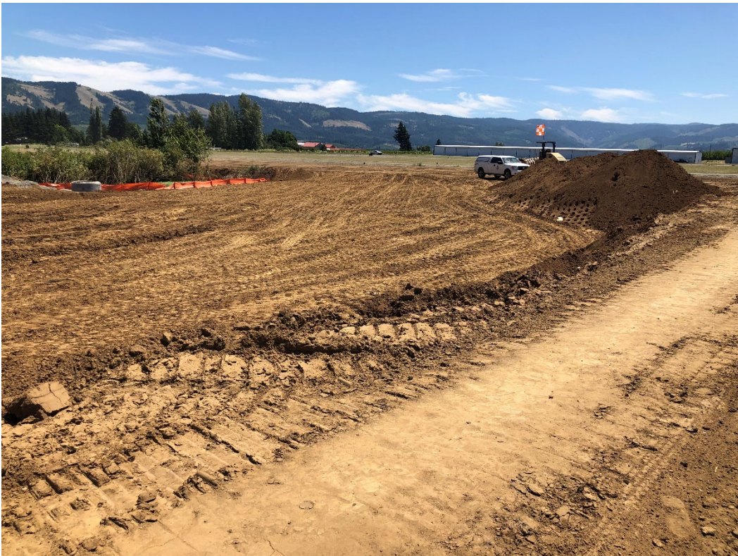
Photo 4. Fill placed in old wetland area within ATERC site. Silt fence in the photo background delineates the limits of the fill and edge of existing wetlands. The sheepsfoot roller (with flag) can be seen behind the fill stockpile.
