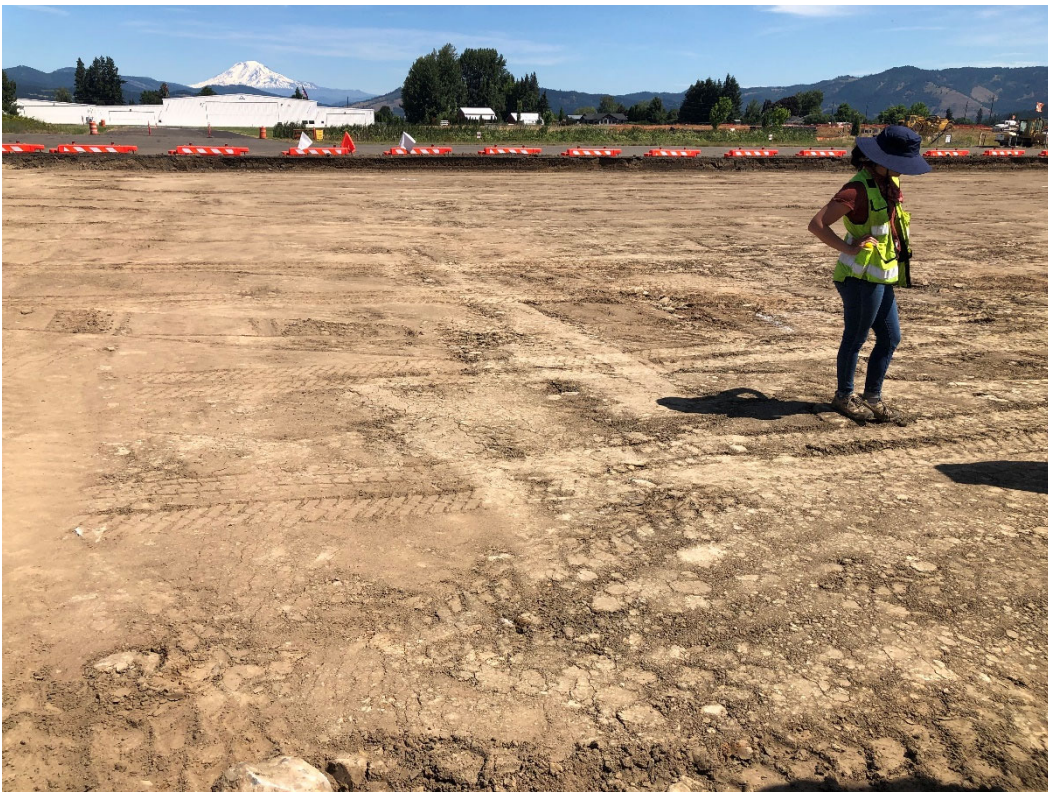
Photo 2. North Apron subgrade at time of proof-roll. Photo taken facing north. Existing, north section of apron can be seen in the background.
