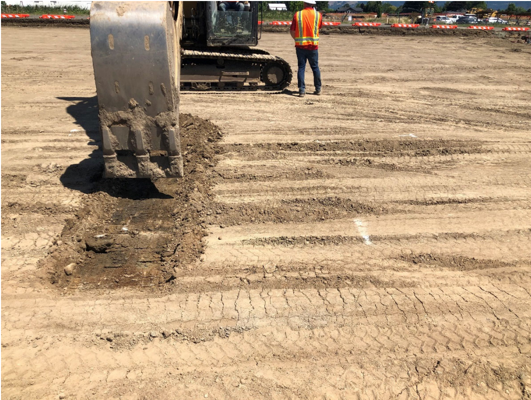
Photo 3. Test pit excavation to observe soils below subgrade surface in North Apron.
