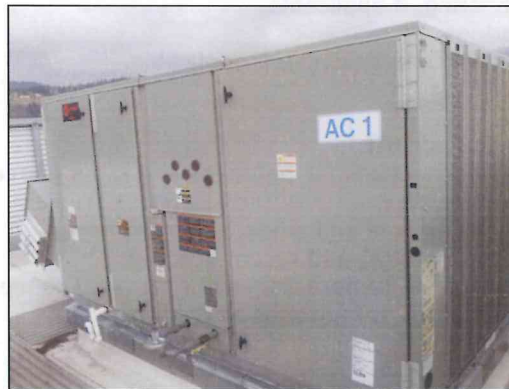
RTU-110: Maintenance- Cooling Season
