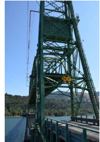
The existing bridge has height and weight restrictions.
