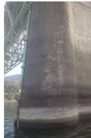
Marine vessel collisions with the existing bridge have damaged bridge piers.
