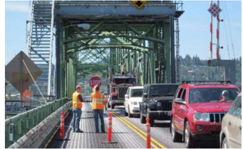
Construction of the build alternatives would reduce ongoing maintenance needs of the existing bridge.
