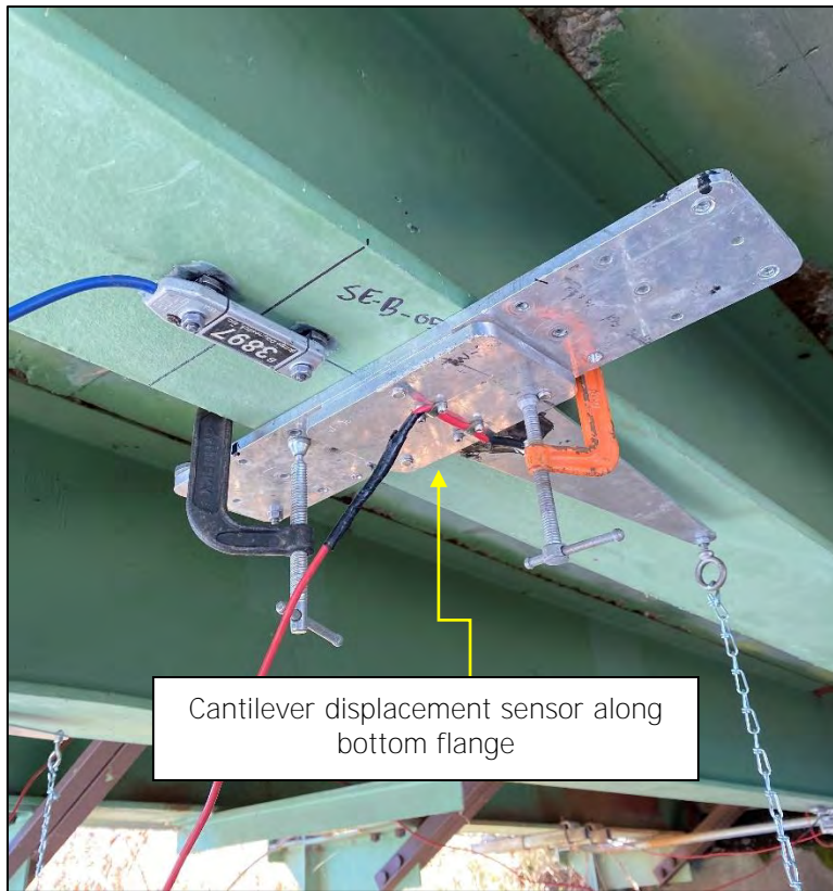
Figure 5 – Displacement sensor along OR approach span stringer midspan (typical)
