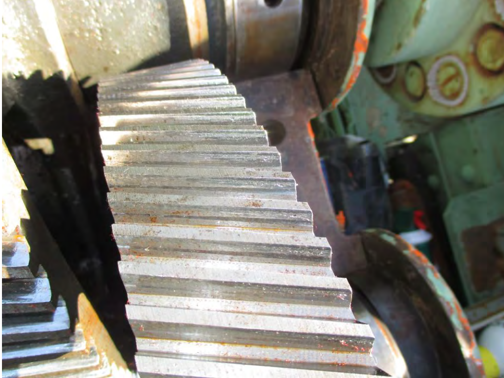
Photo 19. South Primary Reducer. View of east first reduction gear set, opening face of gear teeth. Note the pitting on the outboard (right) ends of the teeth.
