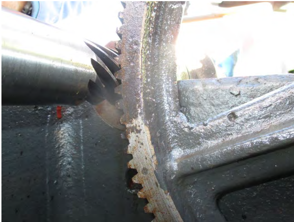
Photo 2. South Primary Reducer. View of the west high speed gear. The side of the gear rim and teeth are corroded.
