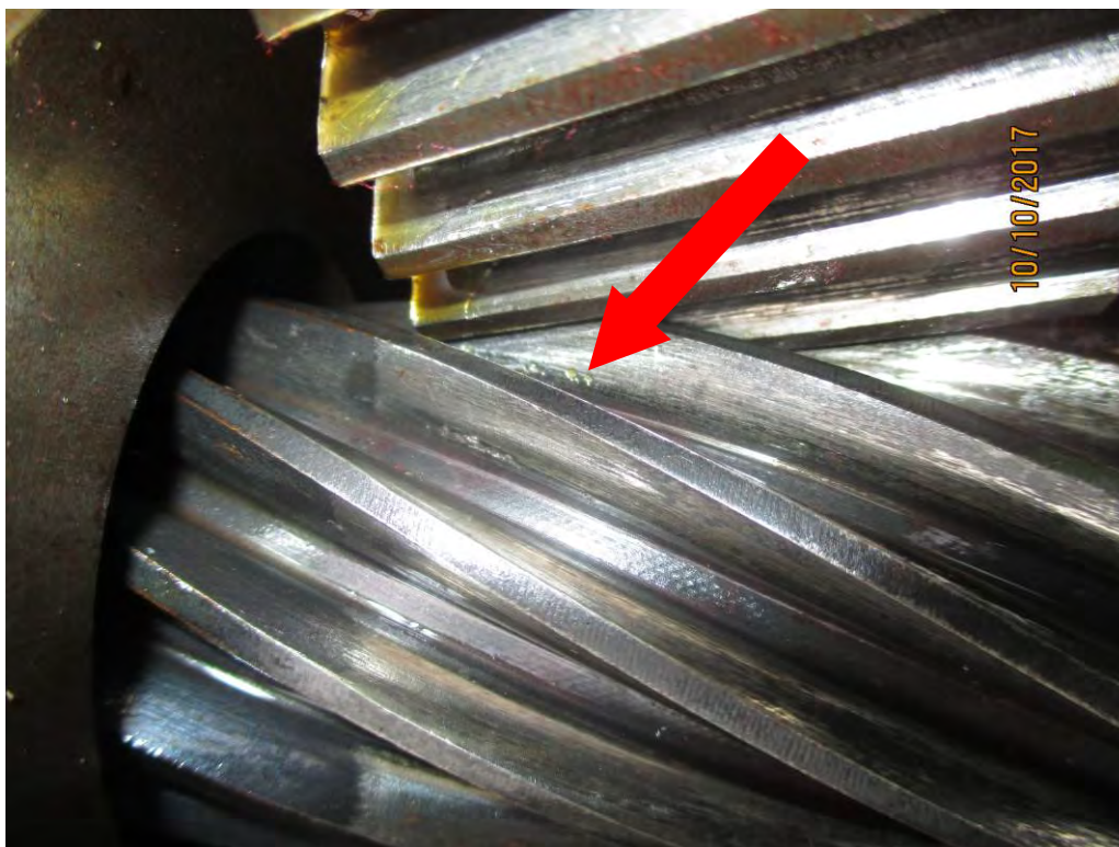
Photo 4. North Primary Reducer. View of east first reduction gear set, opening face of pinion teeth. Note the pitting (arrow) on the east (left) end of the teeth.
