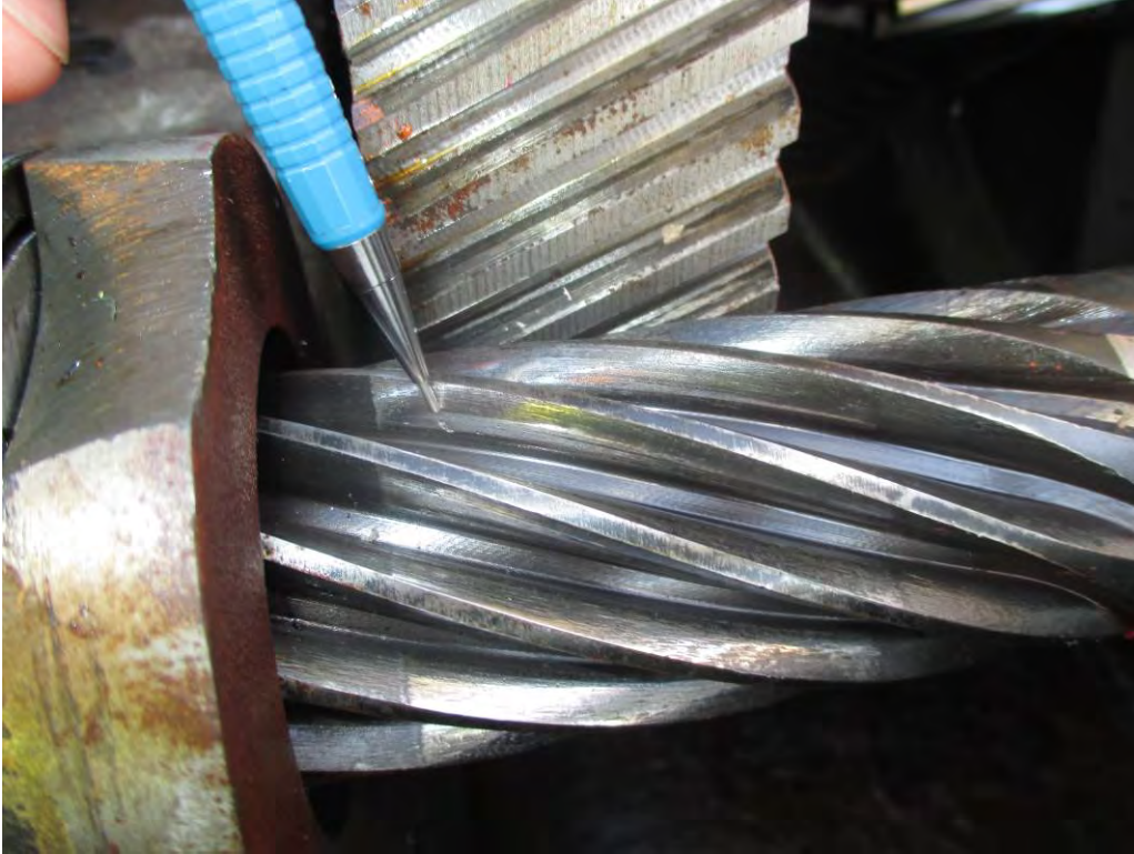
Photo 13. South Primary Reducer. View of west first reduction gear set, opening face of pinion teeth. Note the pits on the outboard (left) end of the teeth.
