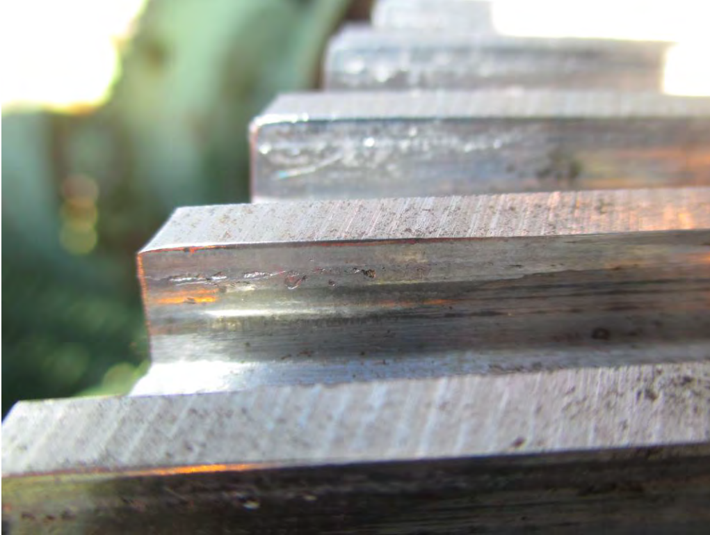
Photo 17. South Primary Reducer. View of west first reduction gear set, opening face of gear teeth. Closeup view of photo 16.
