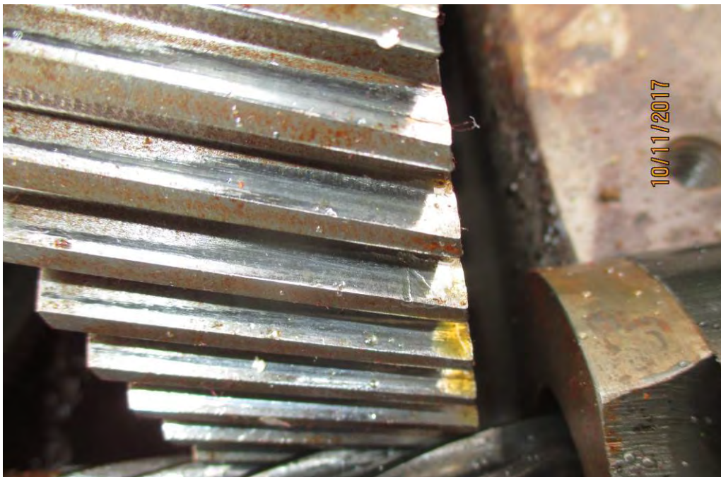
Photo 10. North Primary Reducer. View of west first reduction gear set, closing face of gear teeth. Note the damage on the west (right) ends of the teeth, presumably from particles passing through the mesh.
