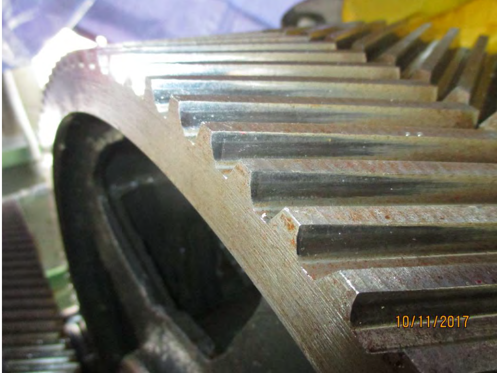
Photo 11. North Primary Reducer. View of west second reduction gear, opening face. Note the contact is 40% to 50% across the width of the teeth, starting at the west (left) end.
