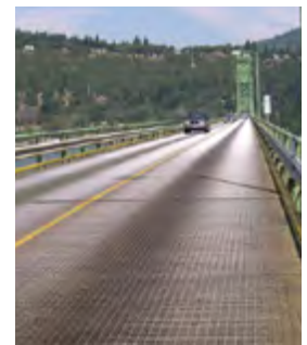
The steel mesh bridge deck is in constant need of repair because of traffic volume and weight.
