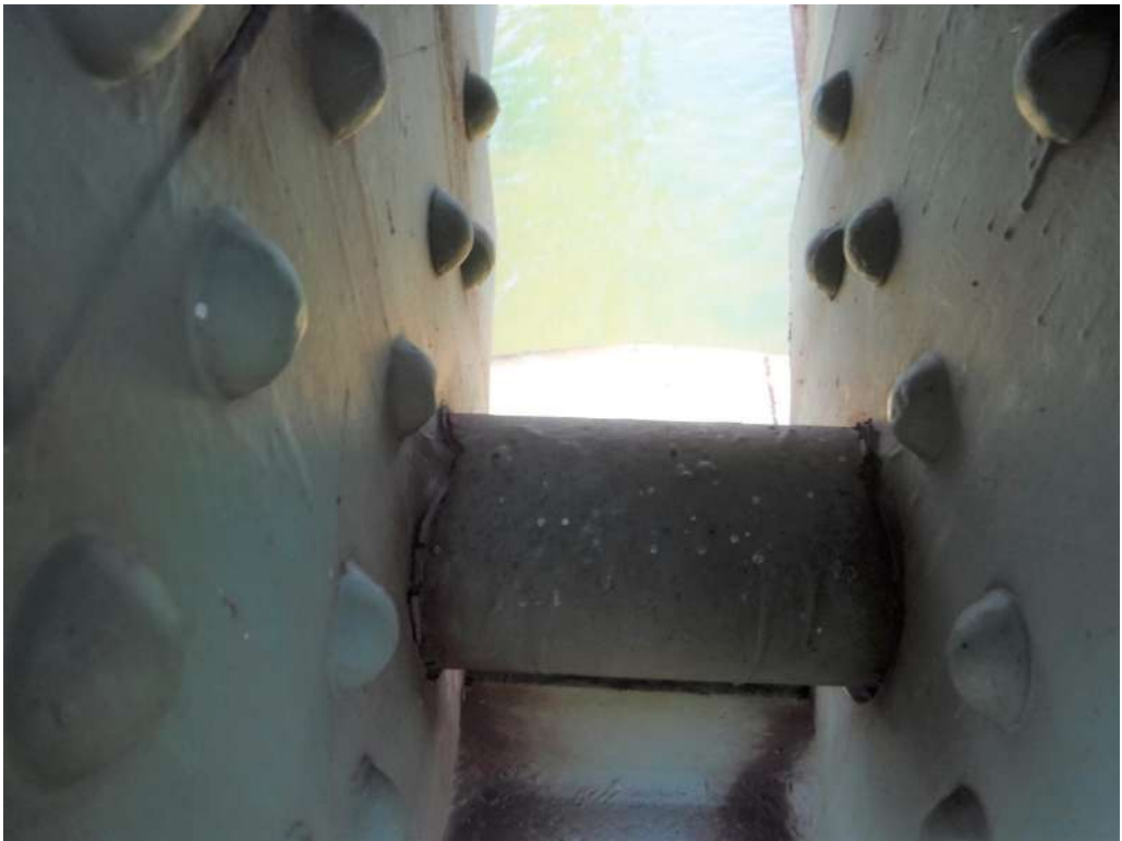
Photo 4 – Bent 19 Upstream Mushrooming
