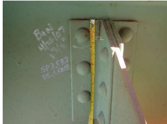
Figure 8. Floorbeam knee brace crack
