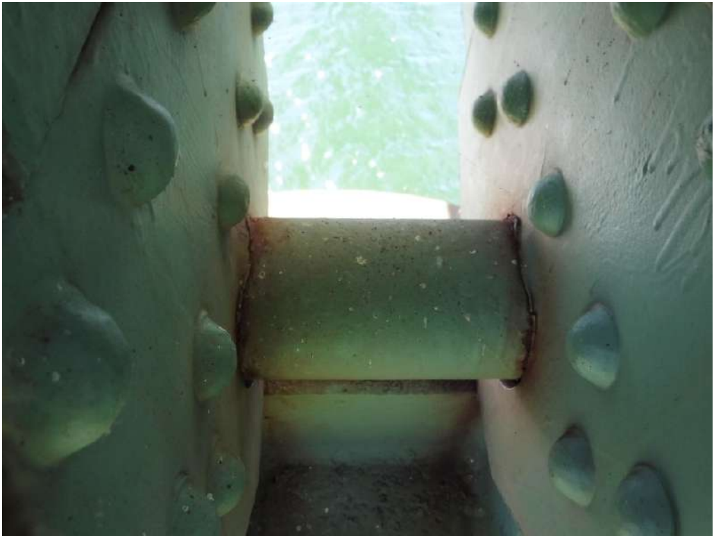
Photo 3 – Bent 18 Upstream Mushrooming
