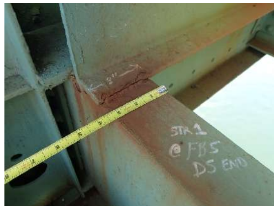
Figure 7. Substringer cracked weld
