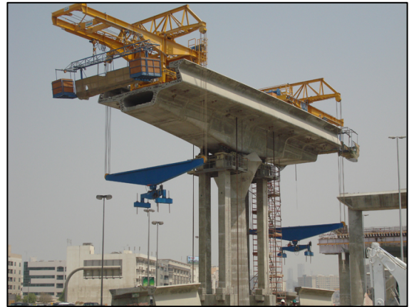
A form traveler used for installing concrete box segments. Use of form travelers is considered out of water work.
