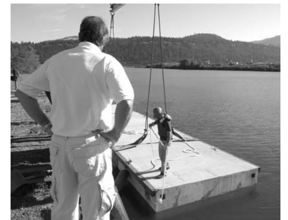
Concrete floats? MSC co-owner Charlie Capovilla looks on to make sure. The 42,000 lb. pier will be used by the company to help build additional larger floats.
