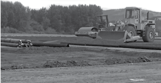
The South taxiways and ramp have undergone a much needed upgrade by Crestline Construction.
