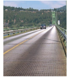
The steel mesh bridge deck is in constant need of repair because of traffic volume and weight.
