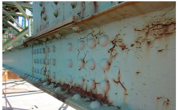
In 2011-12, the Hood River Interstate Bridge underwent the the Lower Chord Rehabilitation Project , a major bridge painting project.
