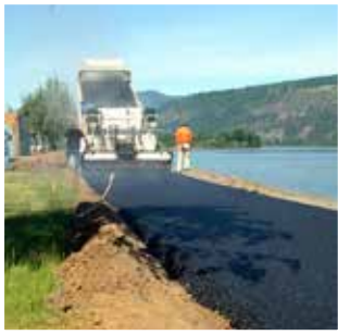
Crews pave a section of the existing waterfront path just west of the Event Site
