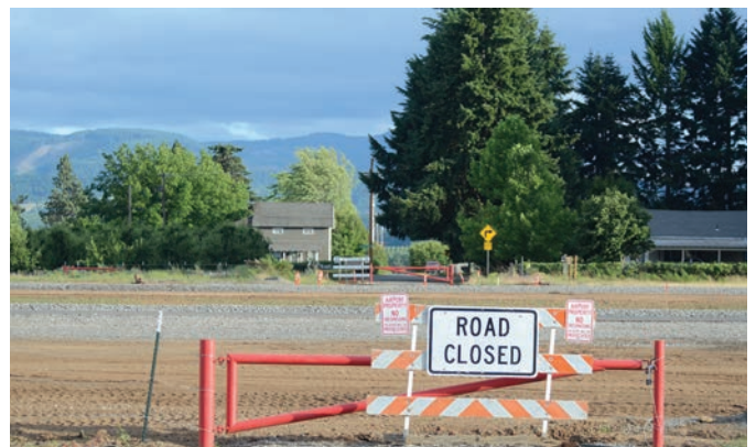
In 2012, the Port completed the Airport Runway Shift, as the first major project of the Airport Master Plan.
