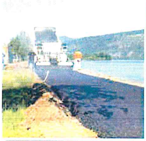
Crews pave a section of the existing waterfront path just west of the Event Site
