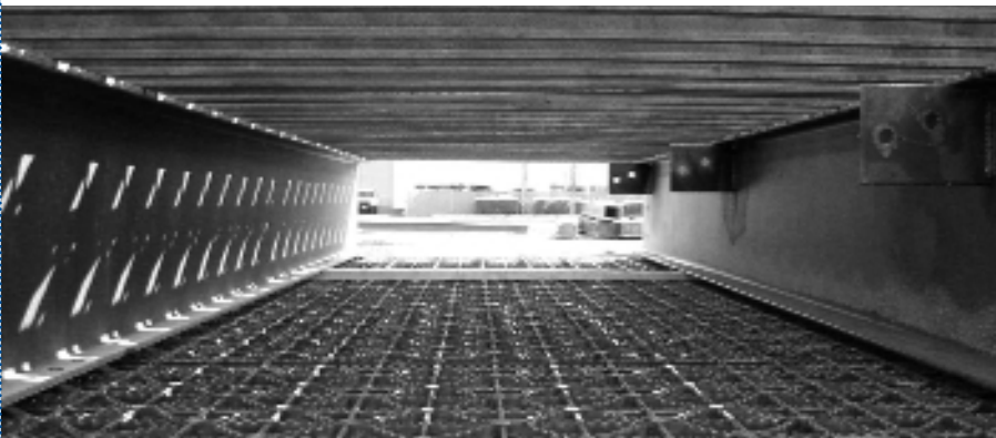
New deck panels are being welded to stringers in Vancouver, Wash., then transported to Hood River. Rail posts will be attached in Hood River prior to placing on the bridge. New guard rails will be the final addition.
