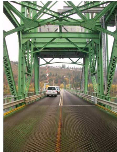
Figure 4. North lift span portal and tower with control house as viewed from lift span roadway.
