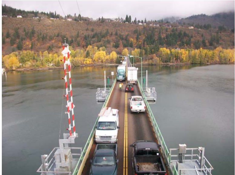
Figure 2. Extremely narrow bridge roadway and steel open grid deck are unsafe for ped/bikes
